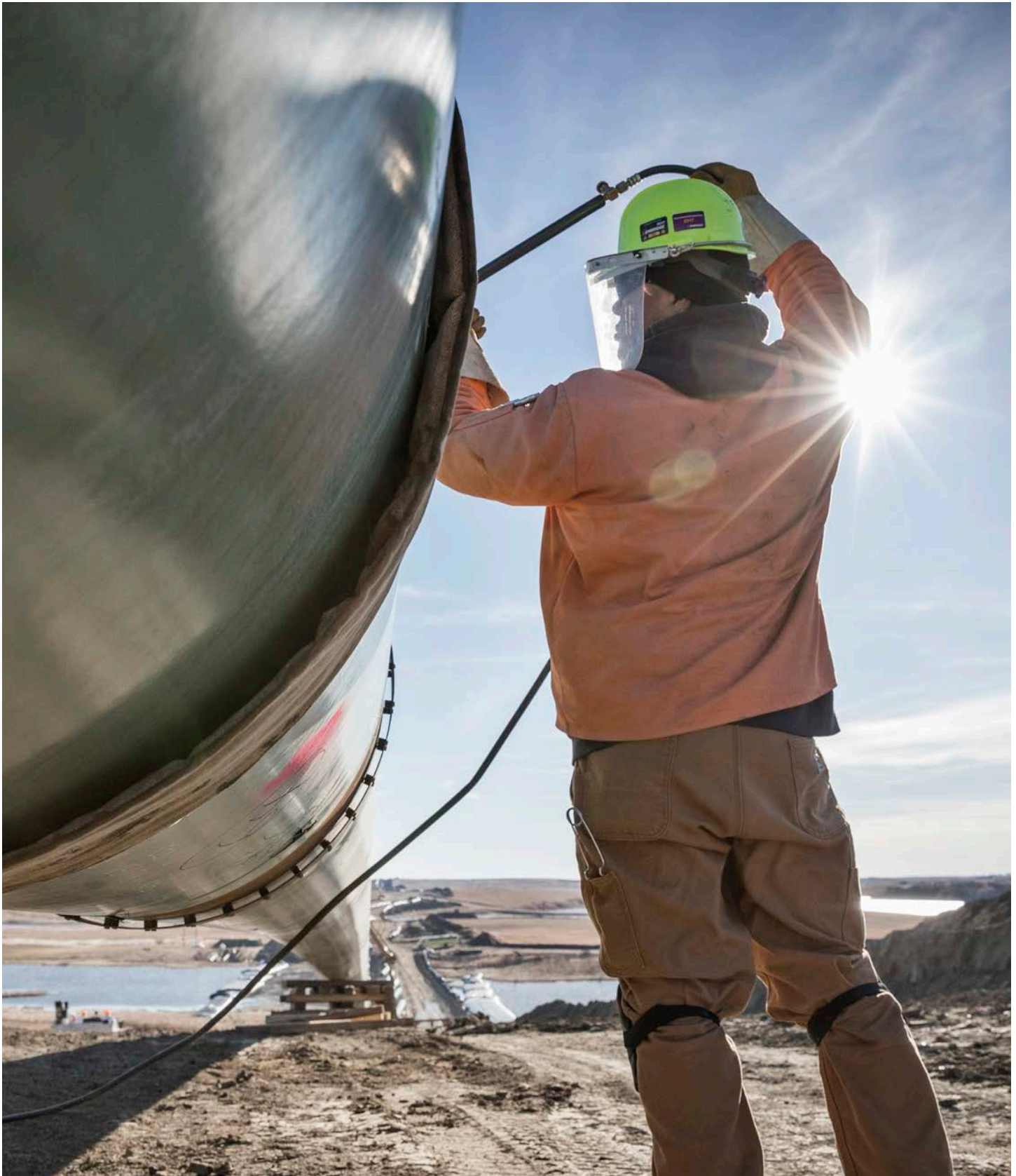
Many workers on the Line 3 Replacement Program in Western Canada are graduates of Enbridge's Pipeline 101 training-to-employment program. Established in spring 2016, this program is designed to teach transferable skills that support future employment opportunities for Indigenous workers across the pipeline industry, as well as related sectors.
