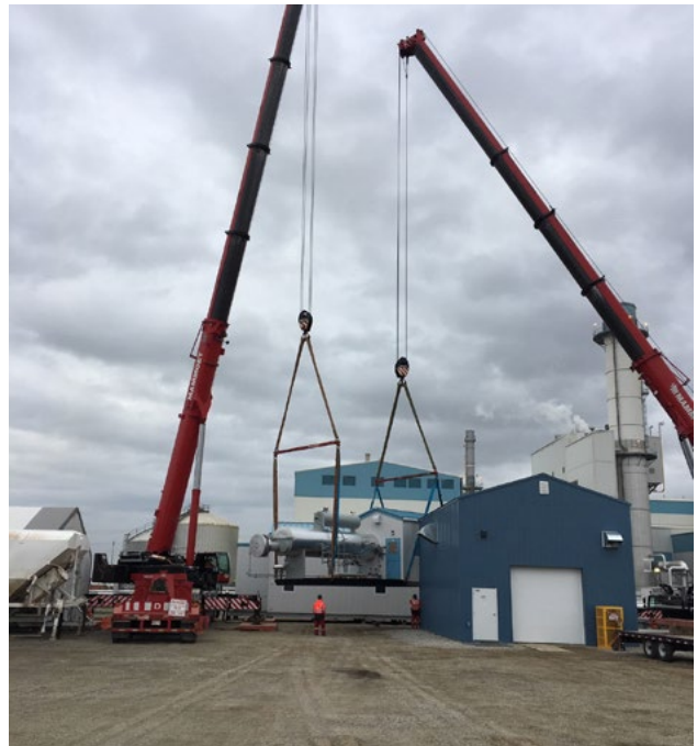
Alberta Carbon Conversion Technology Centre, crédit photo : InnoTech Alberta
